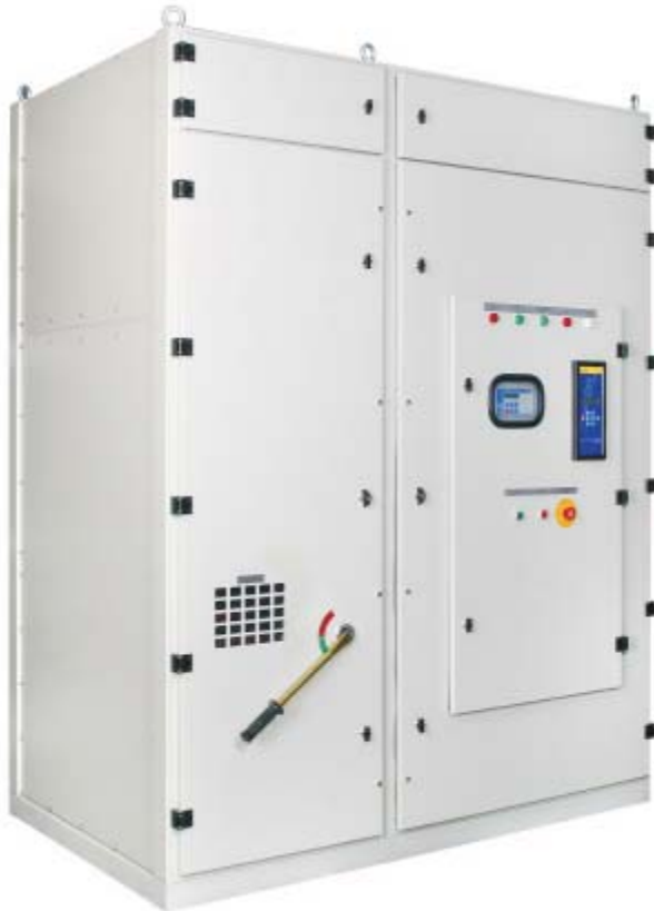
Medium Voltage soft -starter for 3.3KV at 250A. Five units are installed in the Rosh -Pina pumping station.
